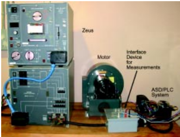
Fig. 3. Test setup for surge testing a motor-and-control system.
