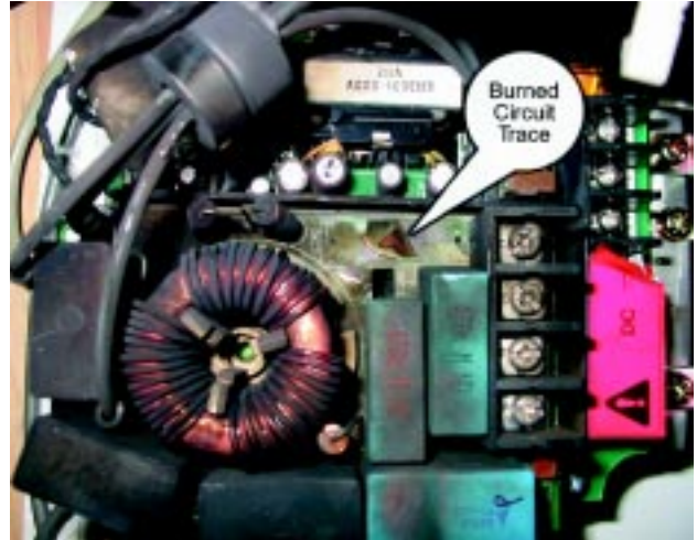
Fig. 6. Damage caused by a surge.
